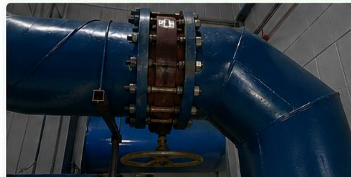
INDUSTRIAL PIPING & VALVES
